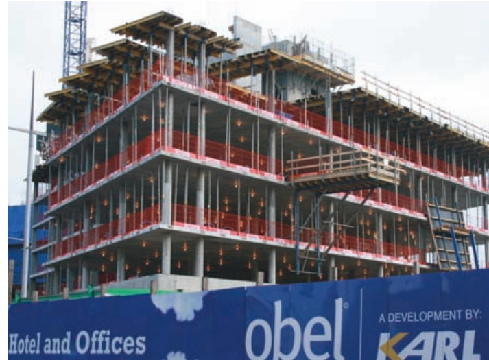
Ridgeway access solutions in place at the Obel Tower development in Belfast.
