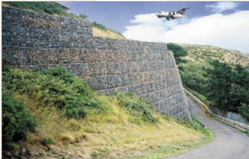
Mass gravity Gabion wall - 19m high and constructed in 1968 to support Jersey airport in the Channel Islands.
