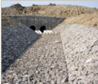
Culvert lining using Mattresses to the A465 heads of the Valley Road, South Wales. Constructed 2004.
